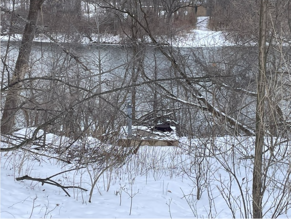
Sewer lift station in northeastern portion of subject property
